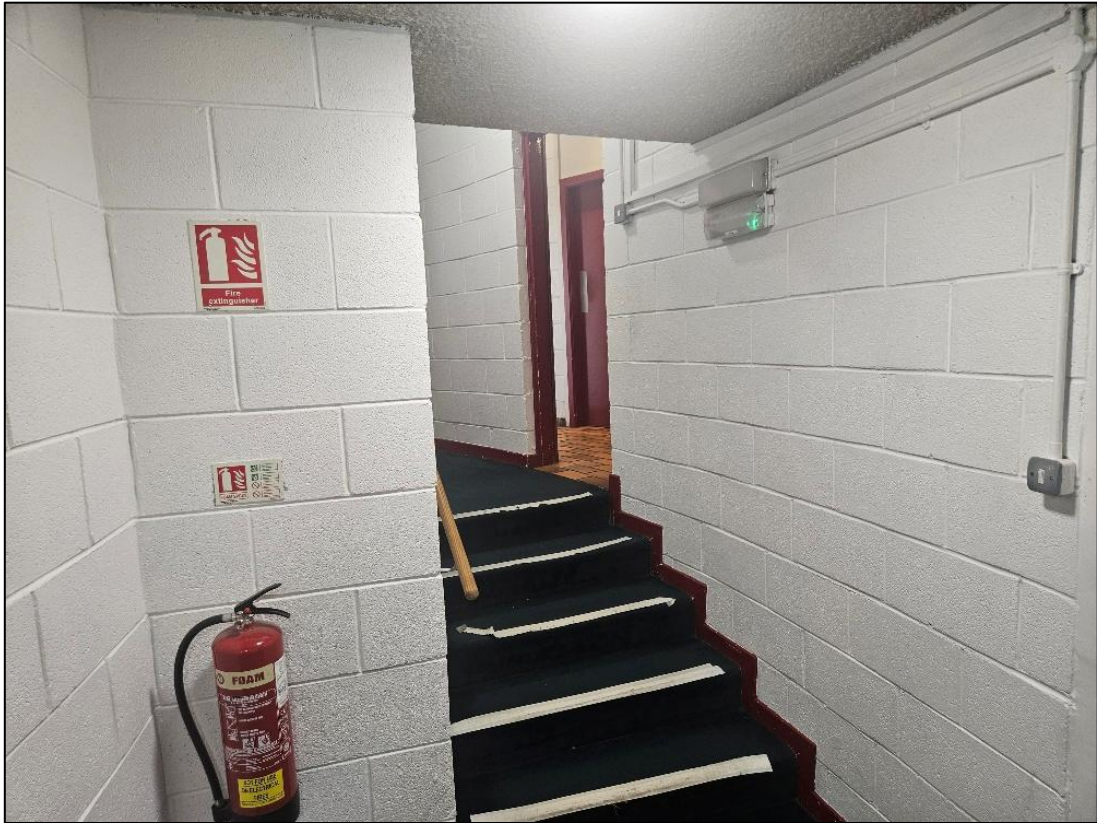
Plate 29 Steps showing the change in level between lower ground and ground floor
