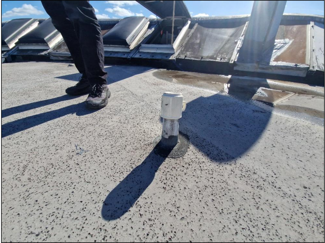
Plate 45 Roof covering and insulation to be addressed
