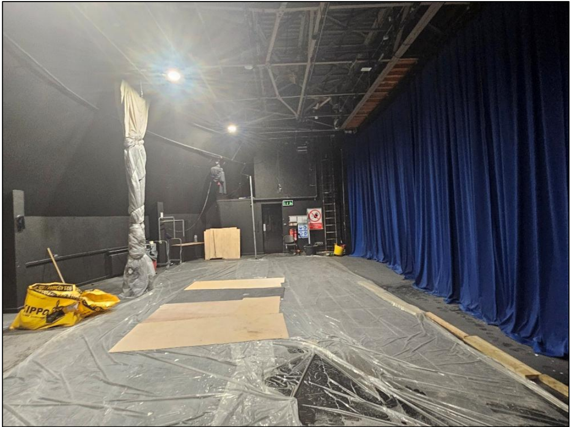
Plate 39 Roof repairs n 2025 will avoid further risks to dancers.
