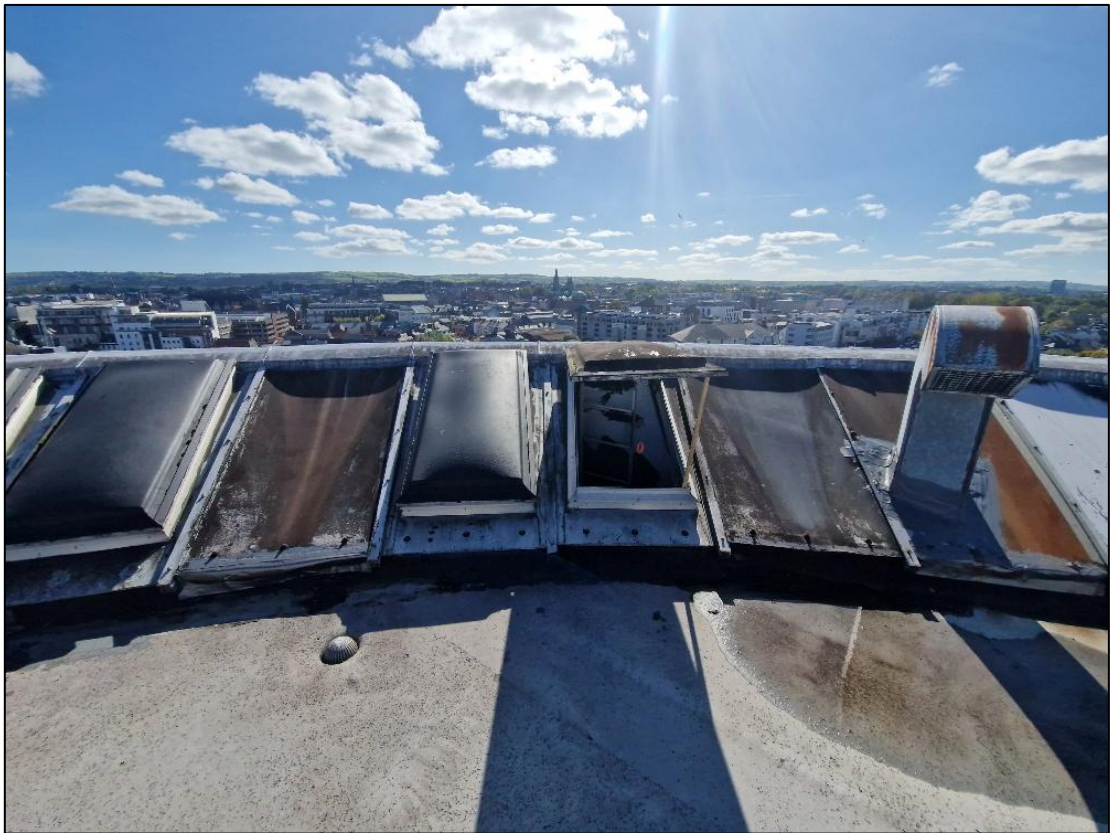
Plate 46 Roof covering and insulation to be addressed.
