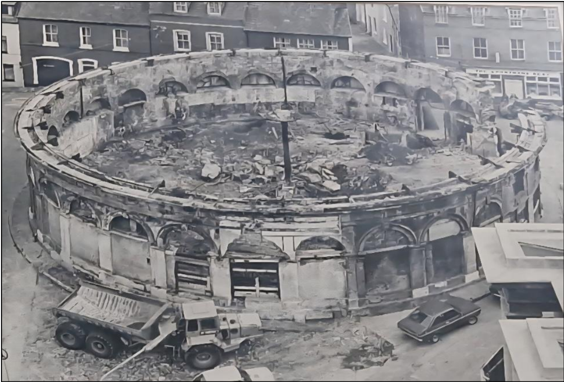
Plate 10 Aerial photograph during the 1980s refurbishment - note central cast iron rain drainage column (c. 24-inch diameter) still standing. Note open arches,
