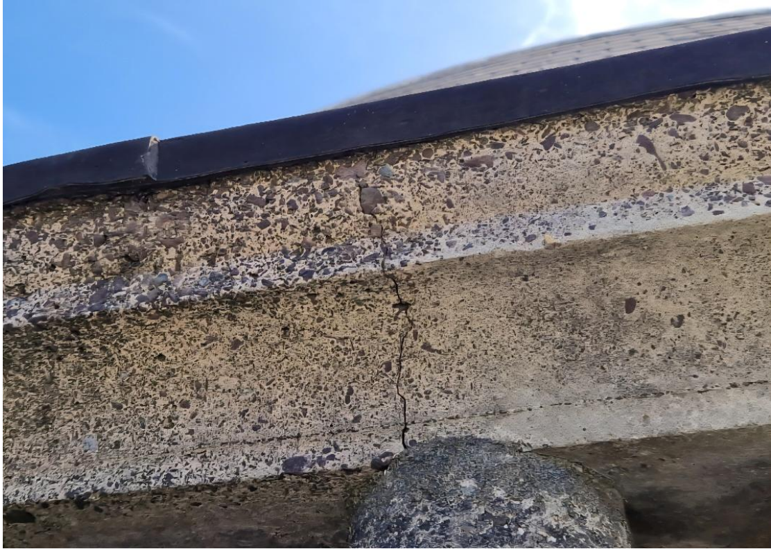
Plate 58 Crack repair and flashing repair are planned for 2026.
