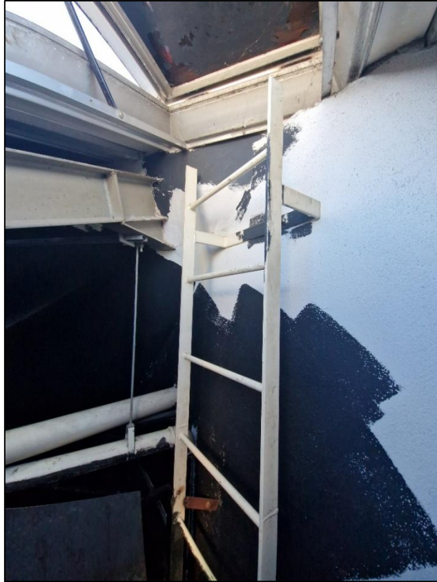
Plate 54 Awkward access to the roof needs to be improved.
