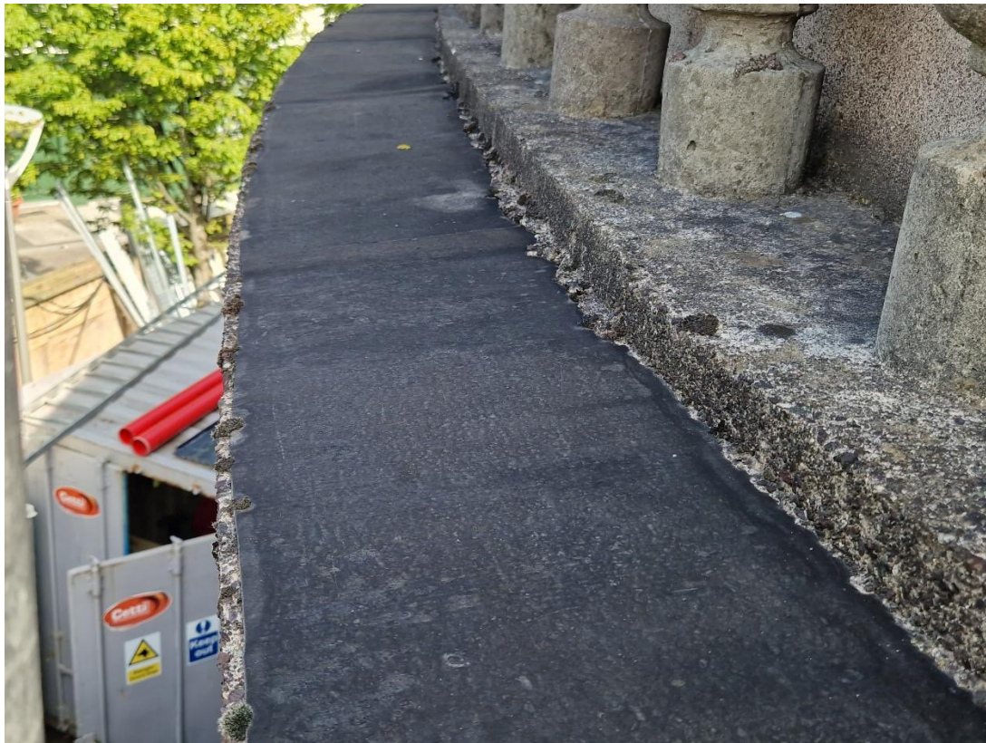
Plate 59 Torch on flashing stops short of the lip edge of the parapet resulting in water staining. To be addressed in 2026.
